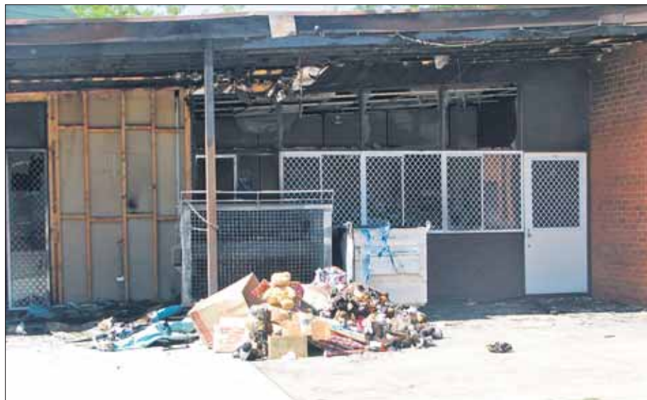
LIMITED DAMAGE: Damage from the fire at St Paul's was limited to one room, despite early concerns that it had spread inside the building. Several boxes of children's soft toys and some clothing made by the Operation Christmas Child sewing group were damaged and had to be discarded.
